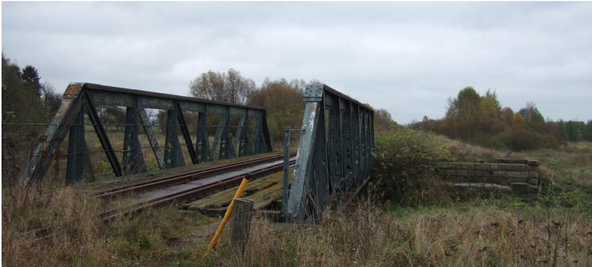
Fig. 1. A view of the railroad bridge at km 25.414 of line No. 30 Łuków- Lublin
