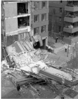
Figure 3. Collapse of balconies in Maastrich
