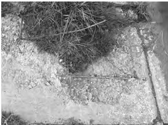
Figure 2. Erosion of surface on concrete slabs (Ageniskis pond) by influence of frost cycles.
