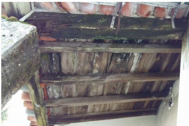
d) Rotting of the timber elements
