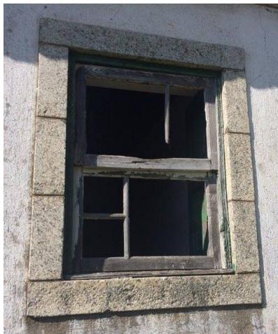
b) Rotting of the elements of wood
