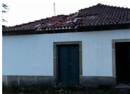
e) Absence and cracking of ceramic tiles
