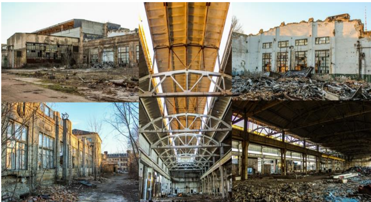
Fig. 1. An example of not functioning industrial facilities in Kyiv city (Kyiv plant "Budshlyahmash") Sources: made by the authors according to the data of the website: URBAN3P Project.
